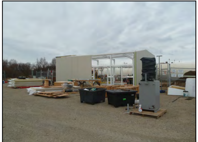
The generator getting a face-lift! The generator has been stripped to the beams & is being completely re-built.
