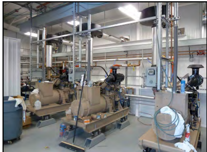
The new generators are turned on & powering the village
